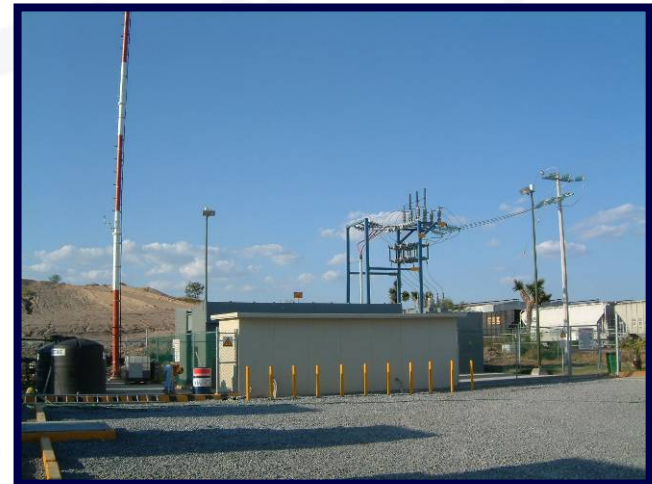
Mexican Landfill Biogas to Energy Plant
